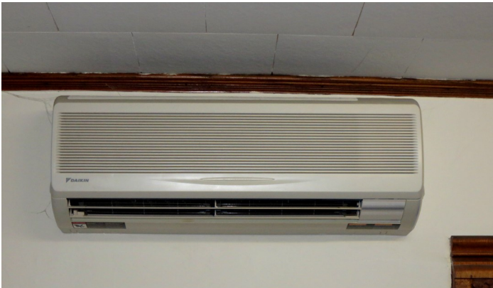
ASHP indoor unit
