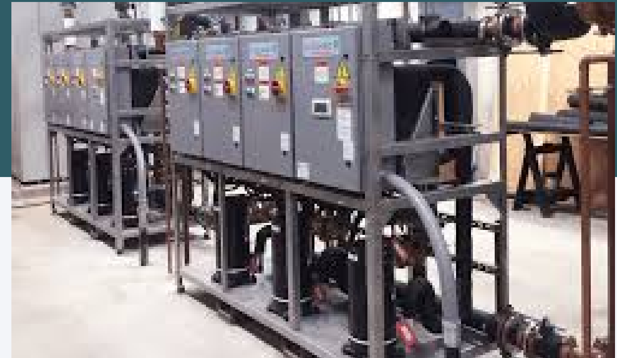
GROUND SOURCE HEAT PUMP
