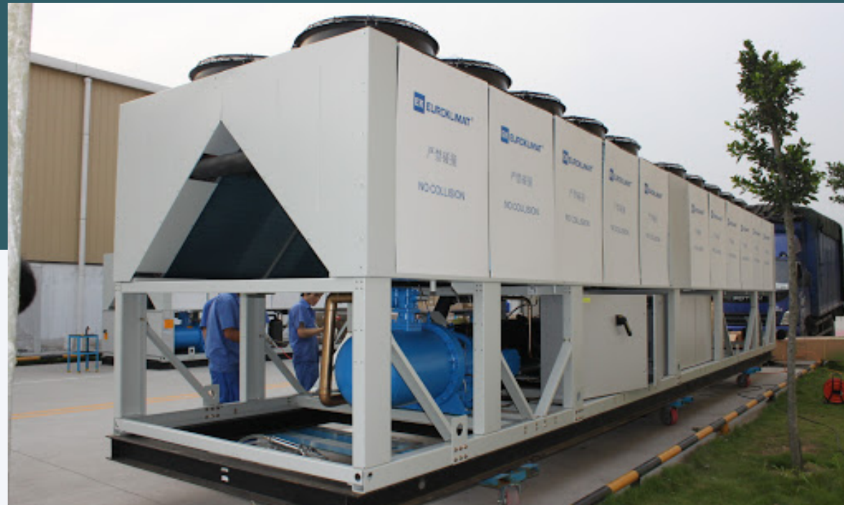
AIR SOURCE HEAT PUMP
