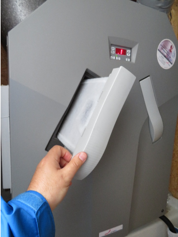
Figure A8. Filter in heat recovery ventilator
