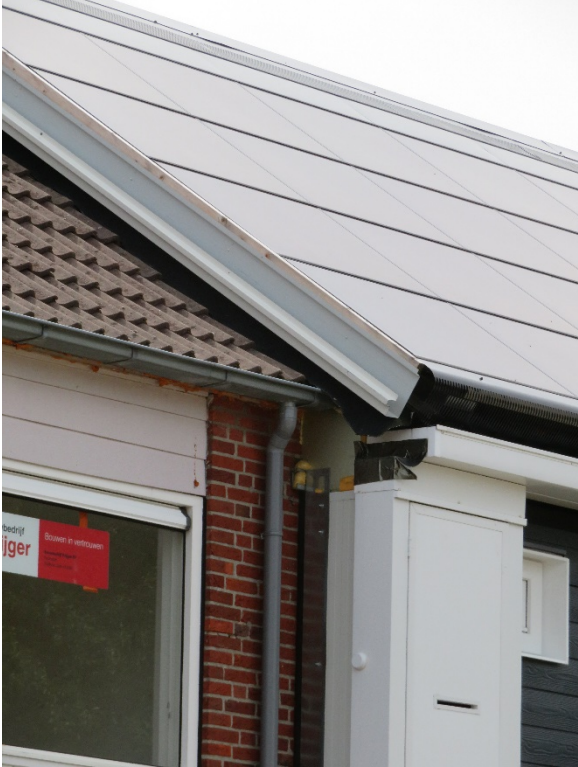
Figure A49. Closeup/detail of not-renovated house adjacent to renovated house
