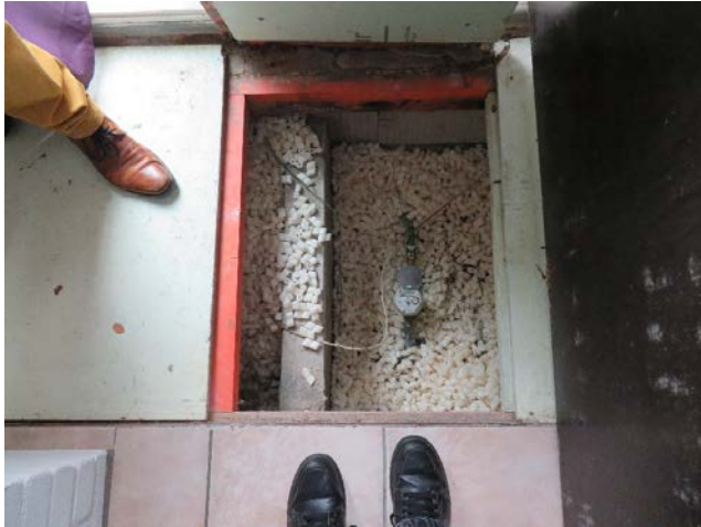
Figure 20. Crawlspace insulated with polystyrene chips
