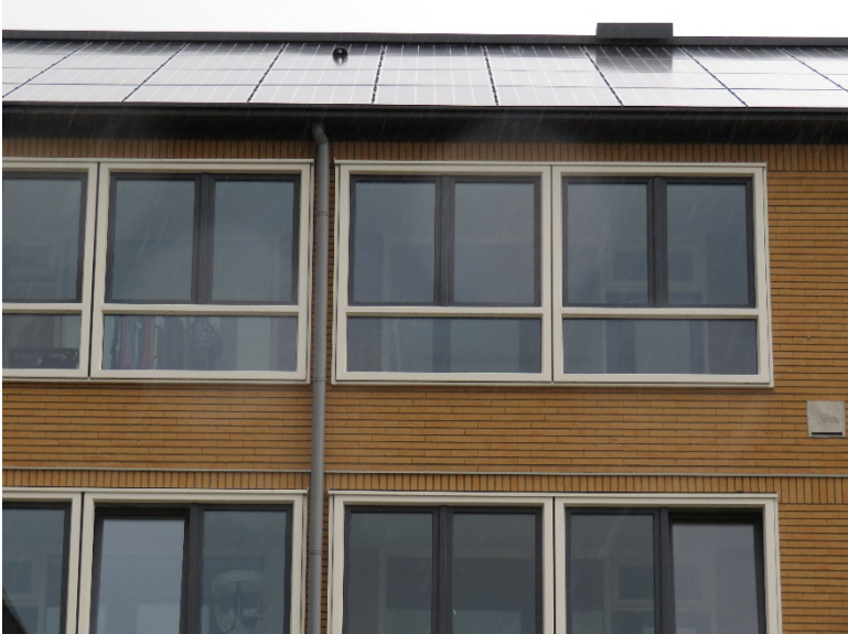
Figure A27. Façade and solar modules on roof on a renovated building
