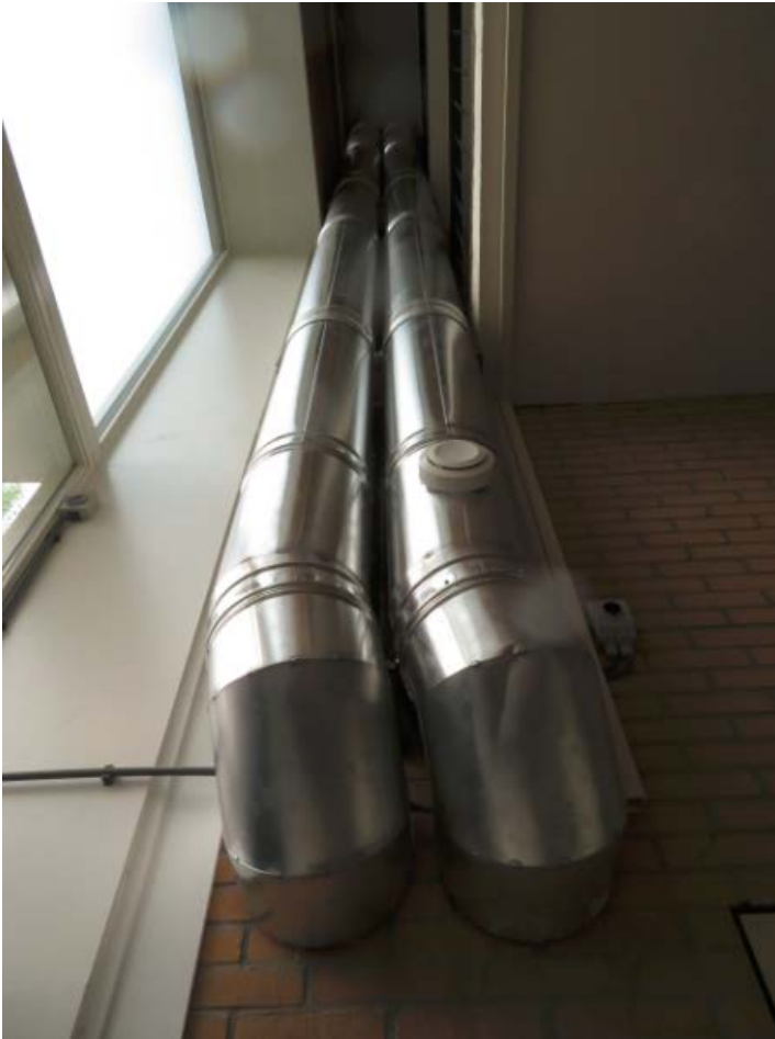
Figure A28. Ventilation ductwork in renovated building
