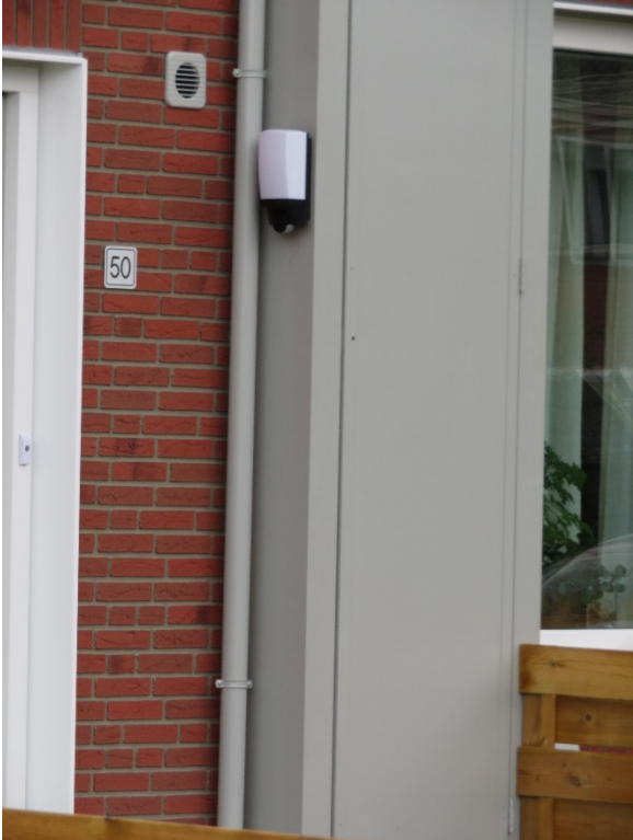
Figure 29. Exterior mechanical enclosure/chase
