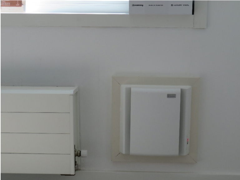
Figure A51. New ventilation fan used on a room-by-room basis
