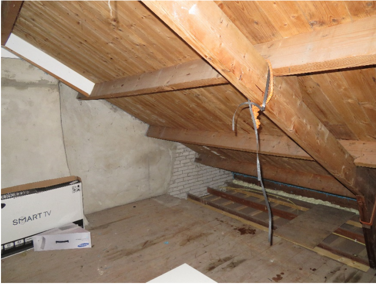
Figure A35. Attic in renovated building showing evidence of air sealing, but insulation is all exterior, above the roof-line
