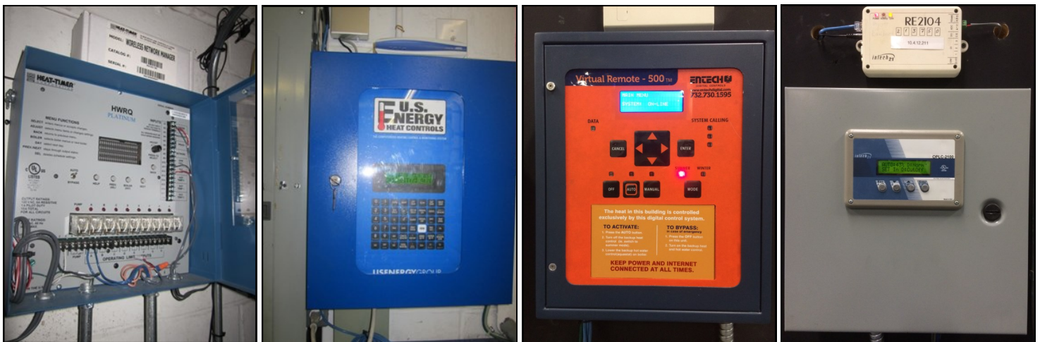
Figure 1: Central computers of Energy Management Systems installed in the field and manufactured (from left to right) by Heat-Timer, U.S. Energy, EnTech, and Intech 21. Photo credits: Far left and left by Taitem Engineering; right and far right by the Association for Energy Affordability.
