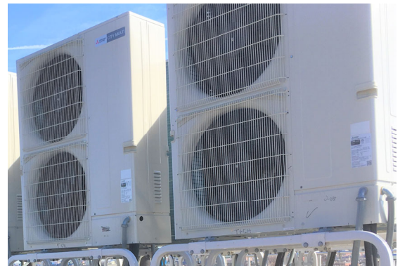
Heat pump outdoor units
