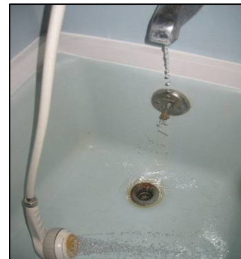
Figure 3: A leaking diverter allows water to flow out both the showerhead and the tub spout simultaneously.
