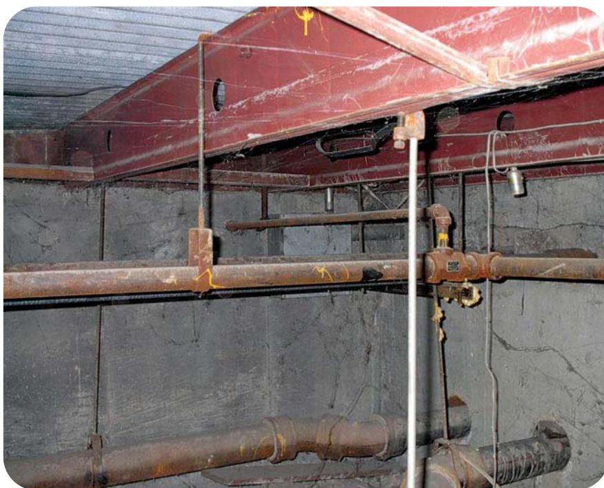
This unimproved crawlspace featured many typical drawbacks, including moisture problems, a dirt floor, and rusty pipes.
